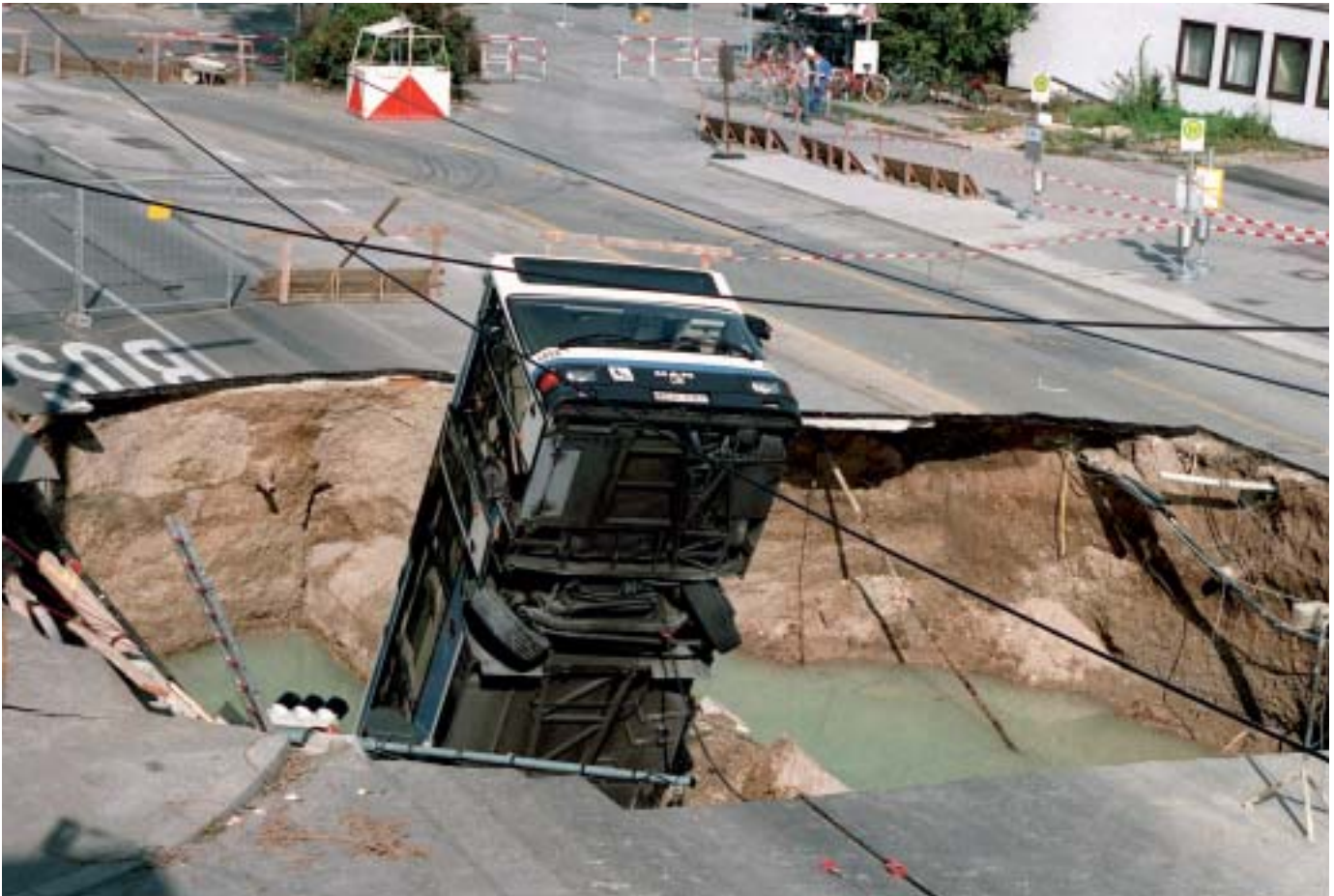
During construction work on an underground tunnel in Munich in 1994, a large crater opened up on a main road, plunging a city bus into a water-filled hole. Three people died and 36 were injured.
